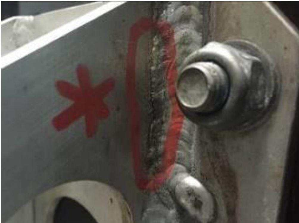
Cracking on a vertical weld – found by DPI
