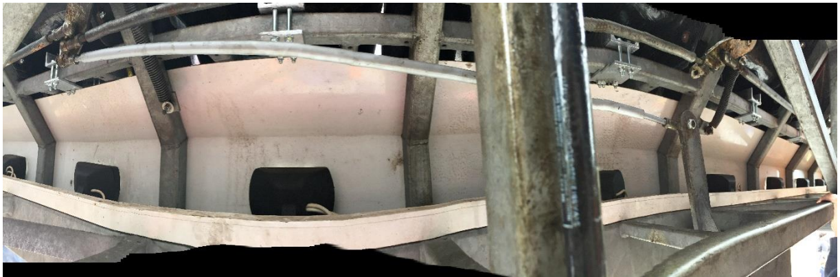
Main adjustment bar to co-ordinate secondary mechanism with primary – note adjustment to right of photo
